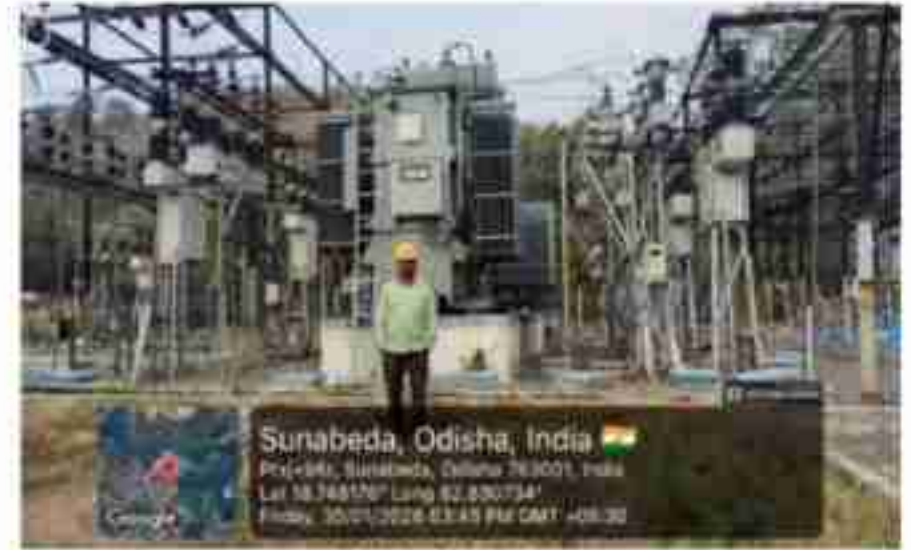
Reliable Power Boost For Sunabeda
